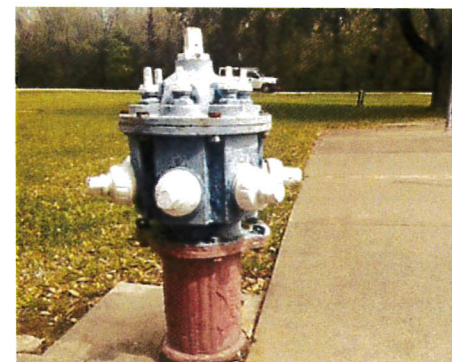
Rare seven-way valve hydrant
